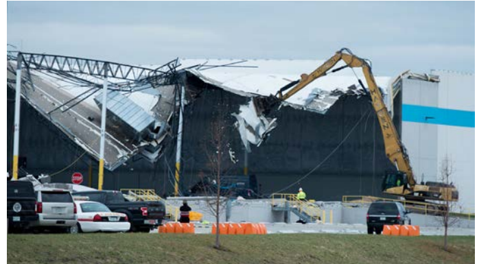
Clearing debris at the Amazon warehouse in Illinois, that was torn apart by a tornado this month. Source: nytimes.com
