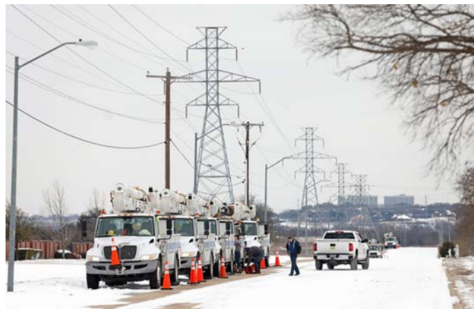
Electric service trucks line up after a snow storm in Fort Worth, Texas, on Feb. 16, 2021. Source: theconversation.com
