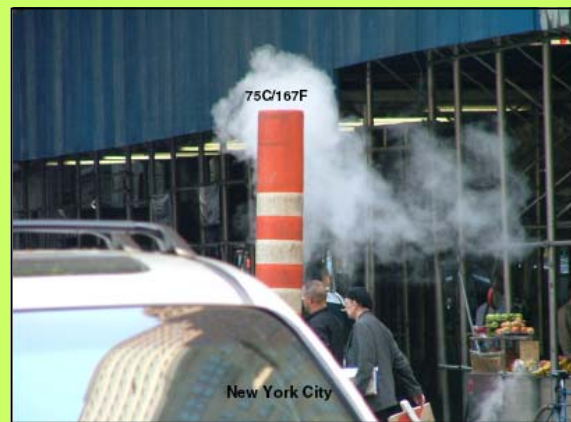
Fig 1. Rooftop and street heat waste in New York. In a summer's day in NYC when the air temperature is 32C, the waste heat at street-level air-conditioner exhausts of CBD buildings is ±58C – substantially hotter than the ambient temperature.
